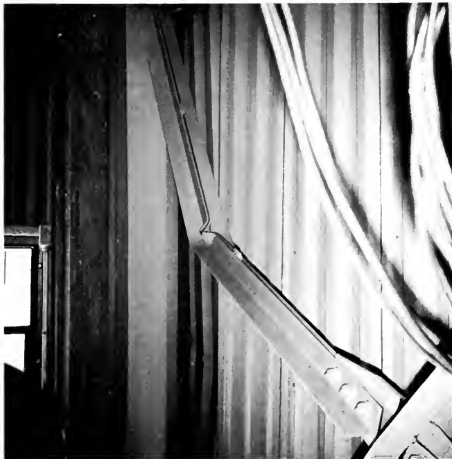
Photo 15. Joseph Jensen Filtration Plant chemical building. Buckled steel bracing member.
